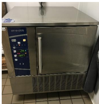
Exterior of Blast Chiller
